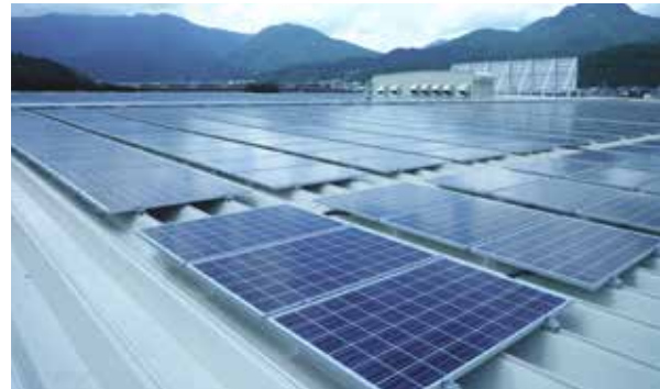
Solar panels at Logistics Center
