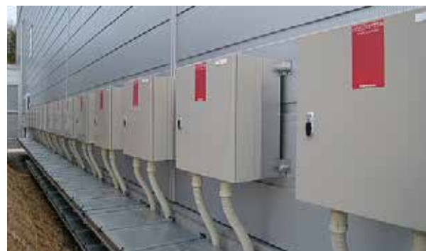
PV Inverters at Fujiyama Works
