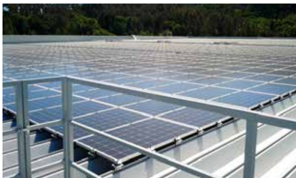
Solar panels at Fujiyama Works
