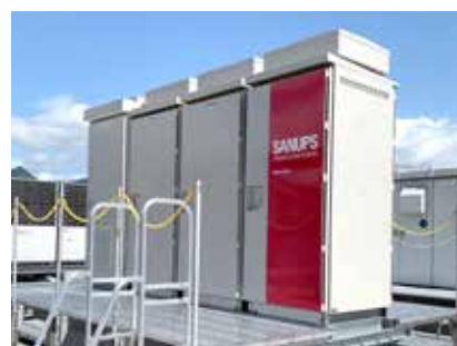
PV inverters at Kangawa Works
